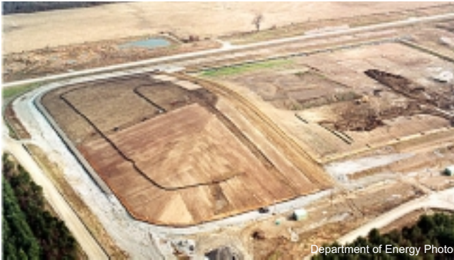
The massive Onsite Disposal Facility at Fernald, in Ohio. Cleanup at Fernald featured local stakeholder involvement and is winding down to most parties' satisfaction.
